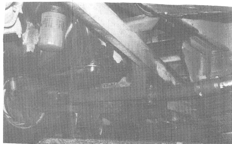
Steel girder motor mount as shown in Craig's #549 V-8. Photo is looking aft.
